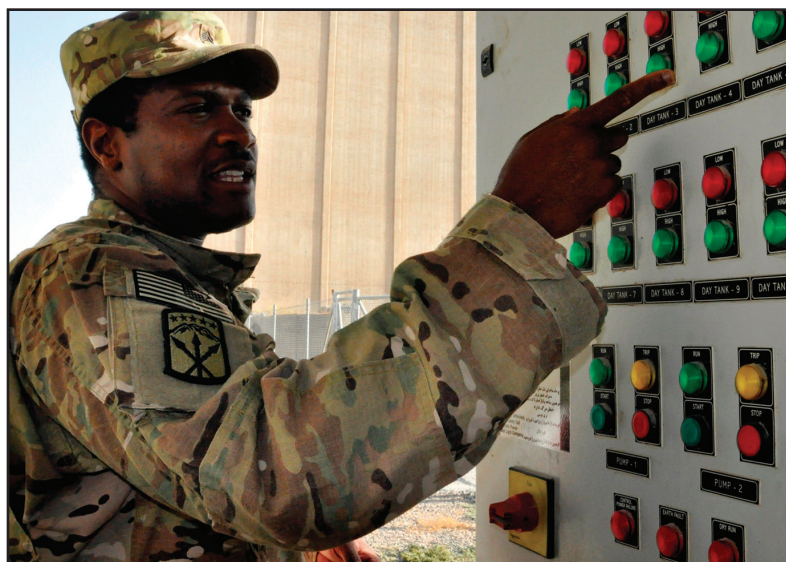
(Photo by Jasmine Chopra-Delgadillo, U.S. Army Corps of Engineers) Sgt. Koutodjo Ayivi, a prime power production specialist and contracting officer's technical representative with the U.S. Army Corps of Engineers' 249th Engineer Battalion, points to electrical equipment 10 August 2013 at the Bagh-E Pol power plant in Kandahar, Afghanistan. The Army faces stiff competition from colleges, other military services, and civilian employers for recruits with the potential to learn complex skills like those of Ayivi.
