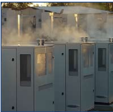
Top: Dyess AFB uses an effluent pond as a cooling tower for the base ice plant, which provides cooling for 14 buildings.
