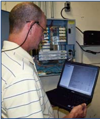
An Energy Management Control System (EMCS) technician at Tyndall AFB configures a Direct Digital Control (DDC) panel to communicate with the EMCS central server. EMCS operators monitor and control building HVAC systems from the server front end.
