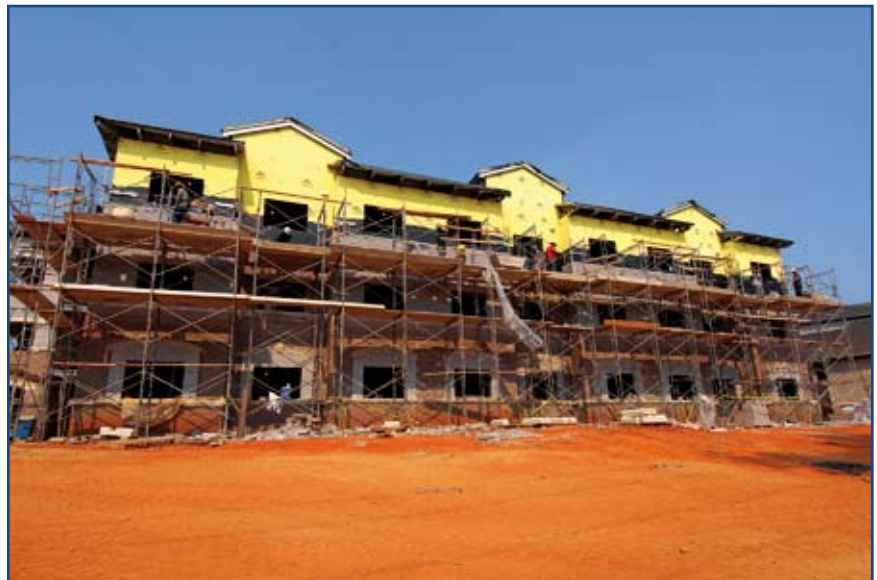
Shaw AFB is investing in environmentally friendly dormitories that are expected to meet LEED Silver certification criteria. One of the technologies in use is a geothermal well for heating and cooling.
