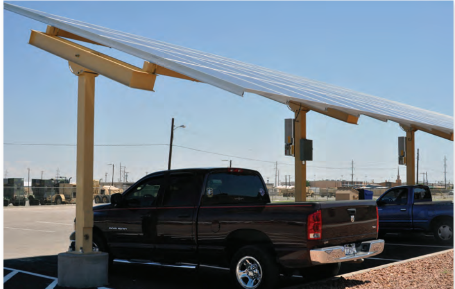
Solar panels used as carports at Fort Bliss, Texas. (Photo by Samantha Reho)
