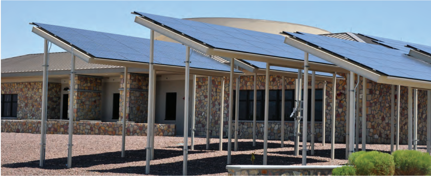
Solar panels at 4th Brigade Combat Team, 1st Armored Division Dining Facility on East Fort Bliss, Texas. (Photo by Samantha Reho)
