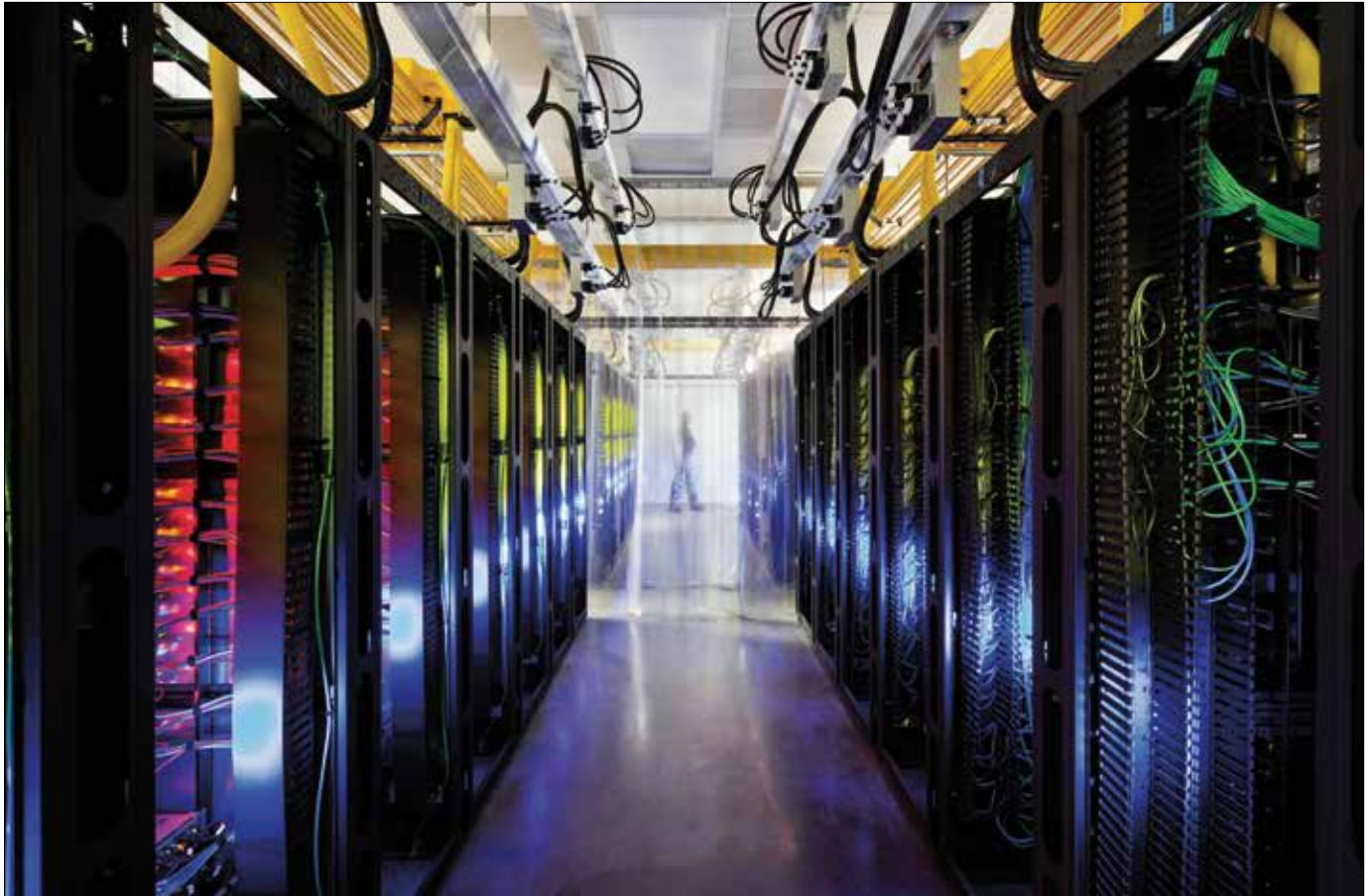
Routers and switches inside Google's campus network room at Council Bluffs, Iowa, allow data centers to talk to one another, with fiber-optic networks that run at speeds more than 200,000 times faster than typical home Internet connections (Photo courtesy Google Inc.)
