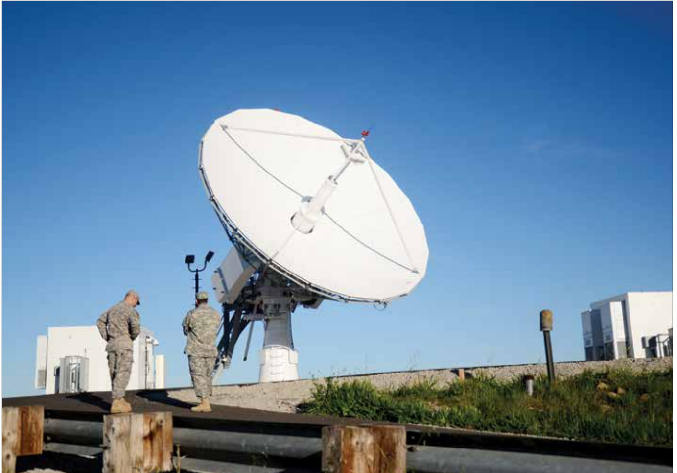
Installation of commercial Internet and phone packages at worldwide regional hub nodes, such as this one in Camp Roberts, California, enables Army and National Guard units to provide commercial services during emergency incidents anywhere on Earth (U.S. Army)
