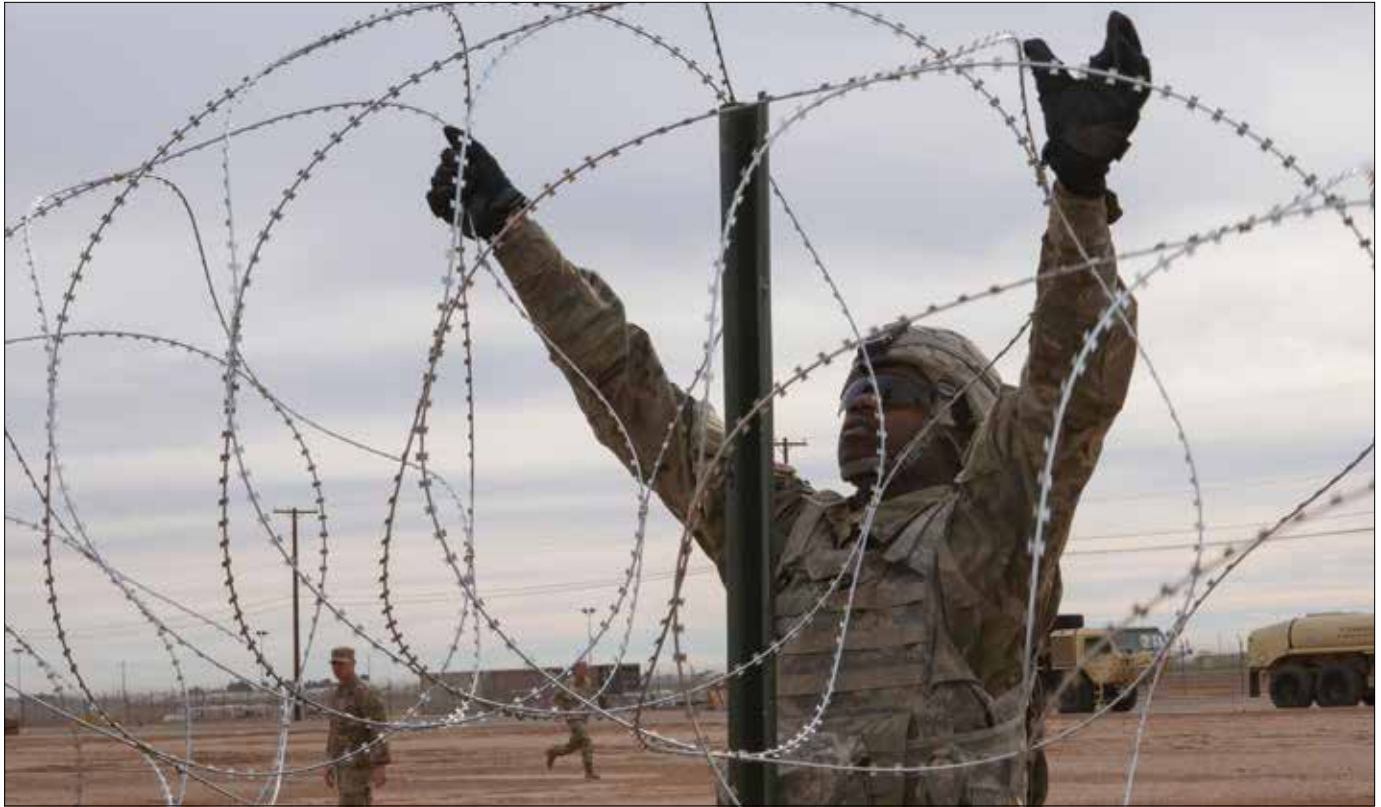
Soldier with 541 st Engineer Company, Special Purpose Marine Air-Ground Task Force 7, moves concertina wire over stake on practice barricade at Naval Air Facility El Centro in California, December 4, 2018 (U.S. Marine Corps/Asia J. Sorenson)
