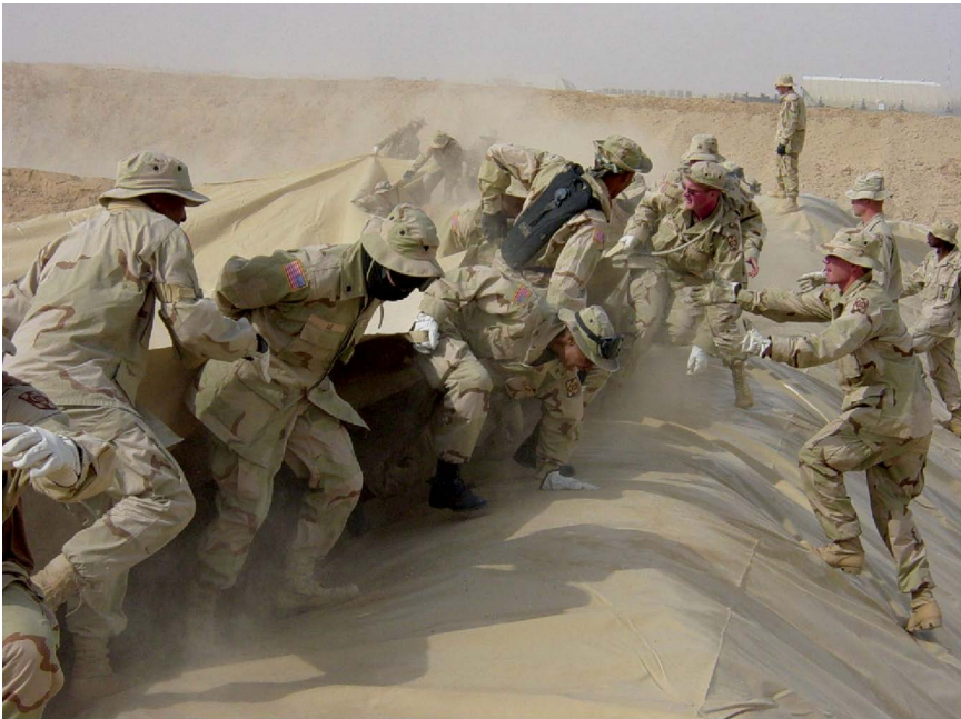
Figure 11.2. Bulk Fuel Tank Assemblies form the storage component of the Tactical Petroleum Terminals that connected the pipeline segments. When combat operations commenced, US forces had more than 4 million gallons of fuel in the TPTs. Photo courtesy of US Army Quartermaster Center and School.
