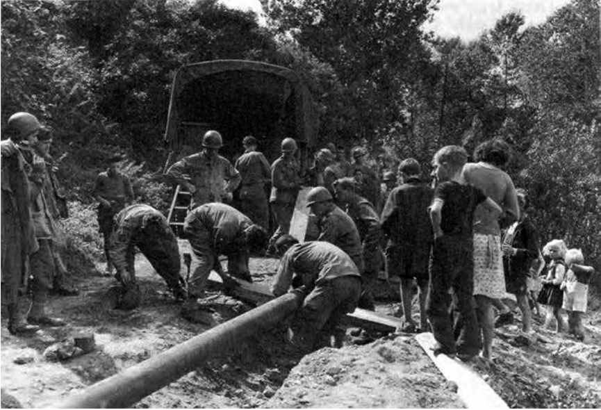
Figure 11.1. The World War II pipeline system consisted of steel pipe that required welding to connect the individual sections. The Army depended heavily on pipelines to move bulk fuel during the war. Photo courtesy of Army Signal Corps.
