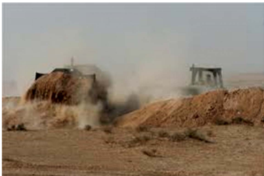
Figure 11.5. To prevent the damage to the pipeline caused by vehicles, engineers constructed 6-foot-high berms on both sides of the line. Ultimately, more than 130 miles of berms were erected. Photo courtesy of 416th Engineer Command.
